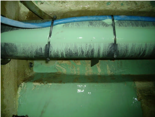
Figure 32: The fans drive shaft is located through the tank and reduces the agitation efficiency.
