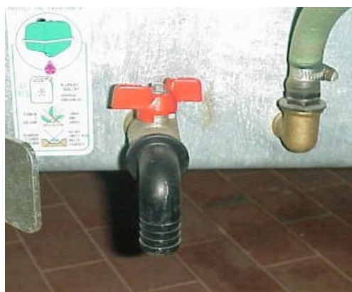
Figure 107: Drain valve positioned at the bottom of the tank.
