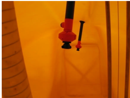
Figure 25: Tank with regular shape where all surfaces can be easily reached by the rinse water spray jet
